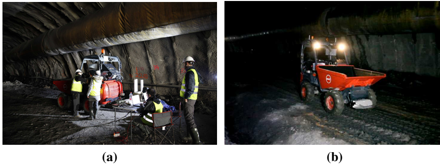
Figure A.14: Experiments with the robotized dumper in the tunnel under construction.
