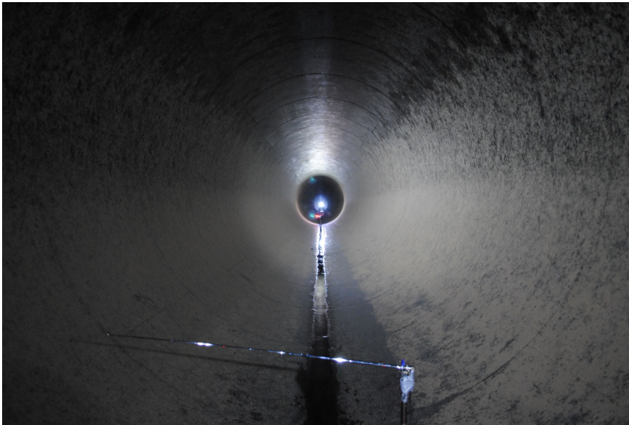
Figure 2.1: Santa Ana dam pipe. Symmetric and smooth inner surface without distinguishable features.
