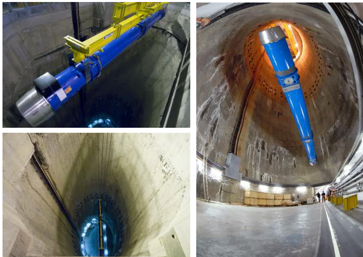
Figure 1.12: The challenge of lowering 1232 dipole magnets to the LHC tunnel. Each dipole weighs 34 tonnes and is 15m-long. Technicians and engineers worked days and nights, carefully installing 20 magnets a week between March 2005 and April 2006. Once they have been lowered down through a single specially constructed shaft, they begin a slow progression to their final destinations in the LHC tunnel, taking about 10 hours to arrive at the furthest point on the LHC ring.
