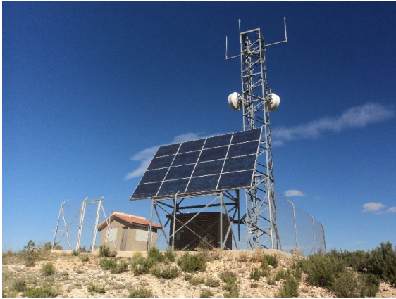
FIGURE 2. PV installation in Morrón, region of Aragón, Spain.
