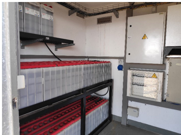
FIGURE 1. Group of batteries of the PV standalone.
