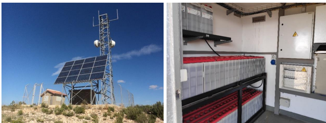
Fig. 4.2. Morrón facility (left) and battery pack (right).
