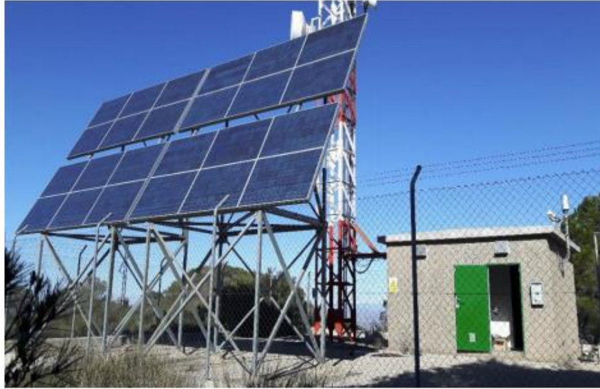
Fig. 1.1. Standalone Photovoltaic Installation in Sigena, region of Aragón, Spain
