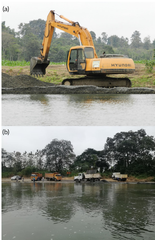
FIGURE 4 Physical destruction of river banks and bottom caused by the removal of gravel for construction. Pictures from the Guayas River basin in western Ecuador
