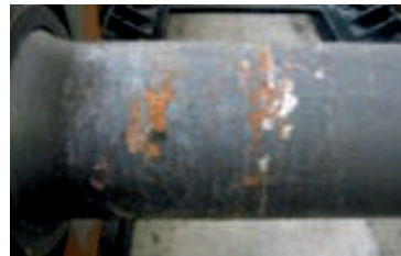
(b) Paint damage and oxidation.
