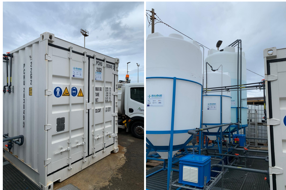
Figure 7. BAoBaB 1 kW prototype installed in Pantelleria island.
