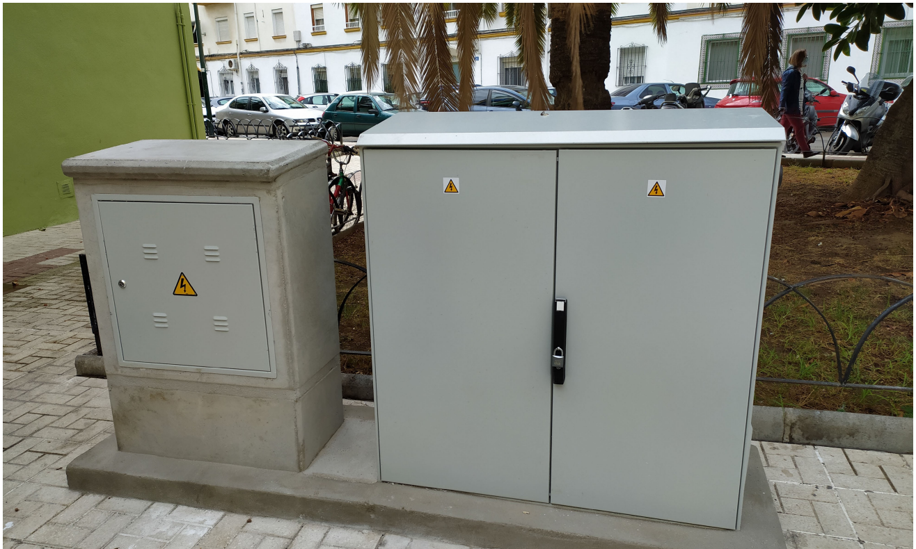
FIGURE 4. D-STATCOM prototype installed in a residential neighborhood in the city of Malaga. The power converter is installed in the cabinet on the right side, while the enclosure on the left side contains the shunt connection of the prototype to the grid, protection elements and measurements of the line downstream of the device.
