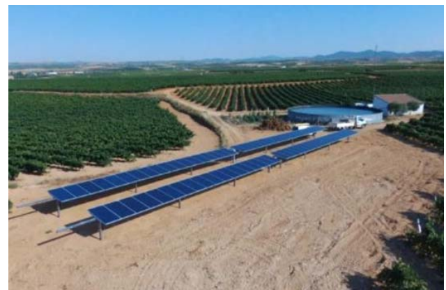
Fig. 1. Installation of solar photovoltaic water pumping for irrigation of a vineyard in Cariñena (Spain).
