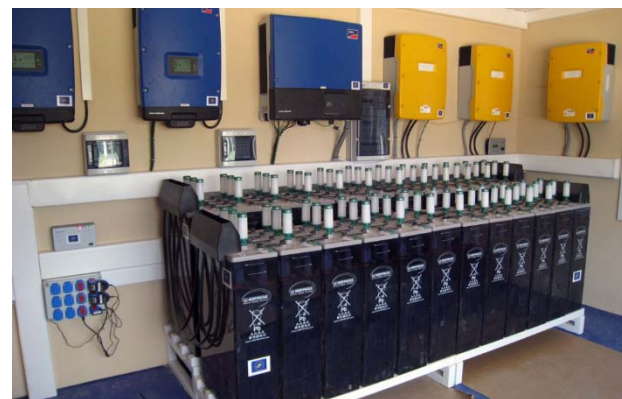
Fig. 3. Batteries and inverters associated with a stand-alone solar photovoltaic water pumping system for irrigation, [13]. Viñas del Vero facility located in Barbastro (Zaragoza); LIFE+REWIND Project.
