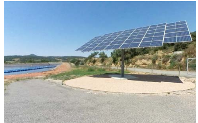
Fig. 4. Photovoltaic panels located on a solar tracker and floating photovoltaic modules. Stand-alone solar photovoltaic water pumping system for vineyard irrigation, [13]. LIFE+REWIND Project.
