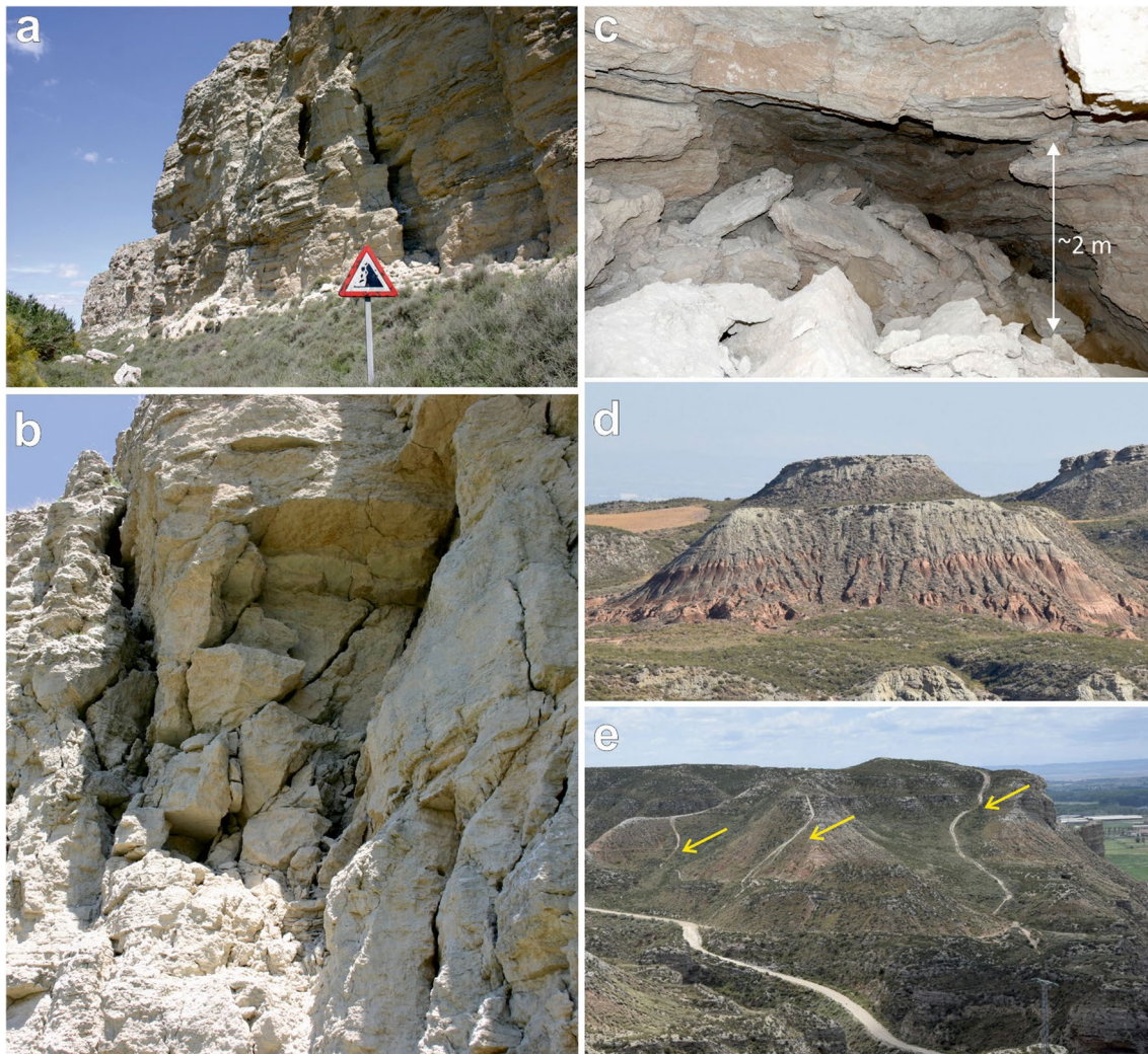
Fig. 18 Examples of geomorphic instability affecting possible developments for geotourism and geo-education. a Strongly disintegrated gypsum cliff at Juslibol, with multiple open cracks. b Close-up of a densely cracked section of a cliff. c Unstable roof and rock debris on
