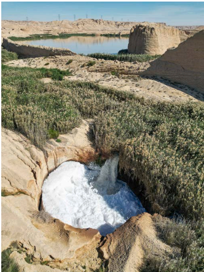
Fig. 25. Collapse in the artificial lake area functioning as a swallow hole with massive water infiltration. The white colour corresponds to turbulence-generated foam from the treated sewage water.
