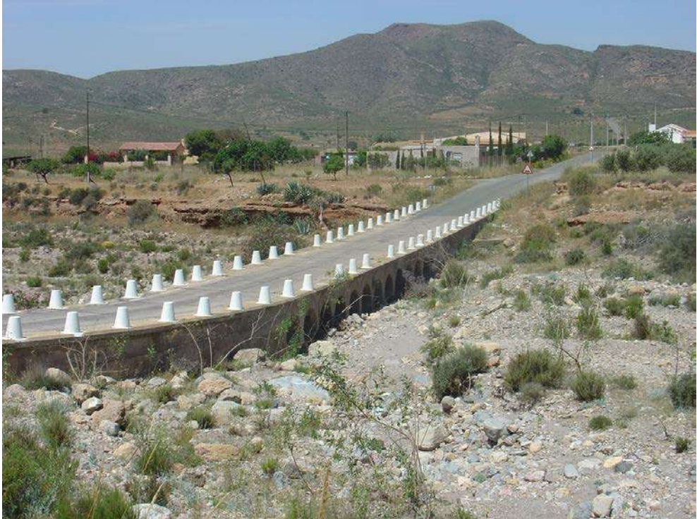
Figure 146. Local road crossing the Rambla de la Azohía (municipality of Cartagena). The culvert-type drainage system, located in this and in so many other road crossings with gravel-bed streams, will have to adapt to the increase in bedload expected for future scenarios of climate change.
