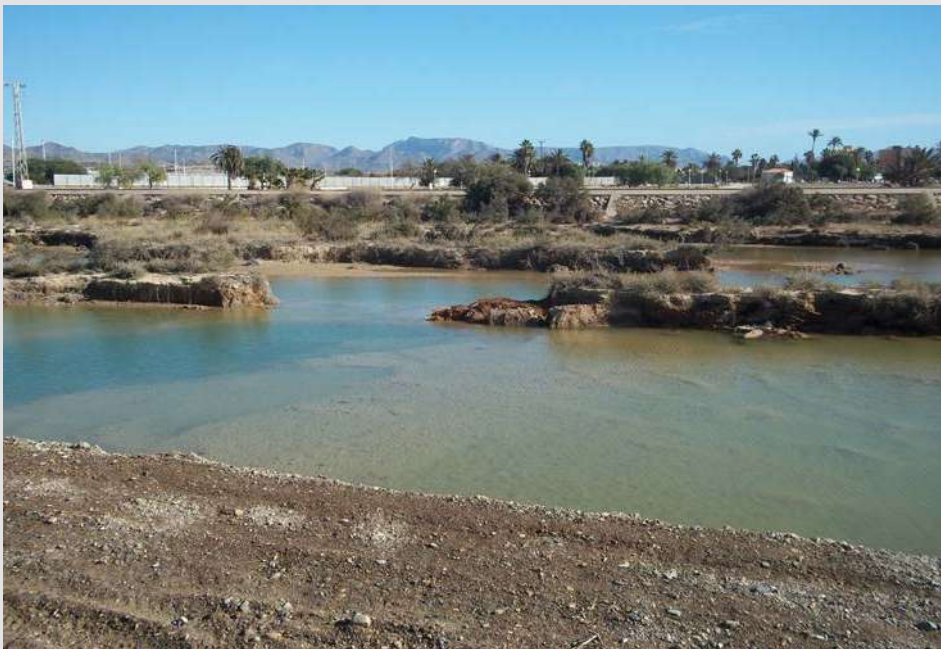
Figures 45 and 46. Dredging and removal of sediment from the Rambla de las Moreras (Mazarrón, Murcia) in its final reach, affected by incision.
