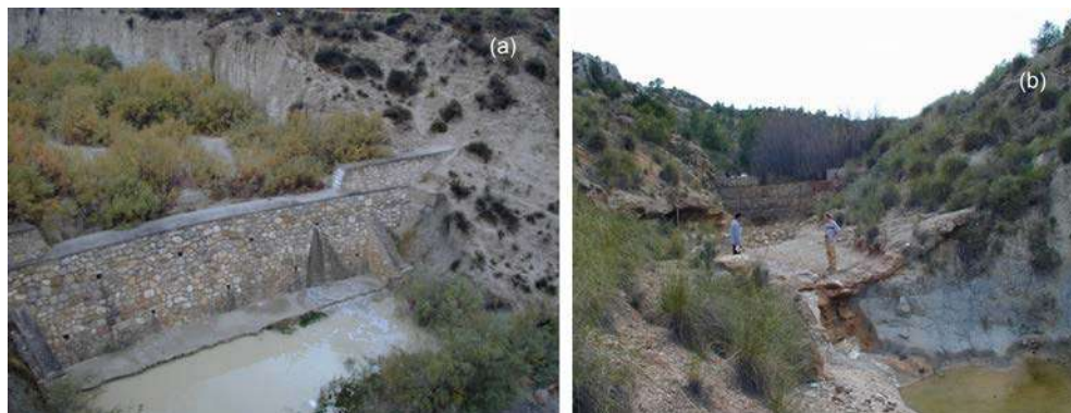
Figures 140 and 141. Masonry check dams installed in the basin of the Rambla del Cárcavo in the lower (a) and middle reach (b) (Cieza), responsible for heavy surface washing, silcrete formation and bed erosion downstream.
