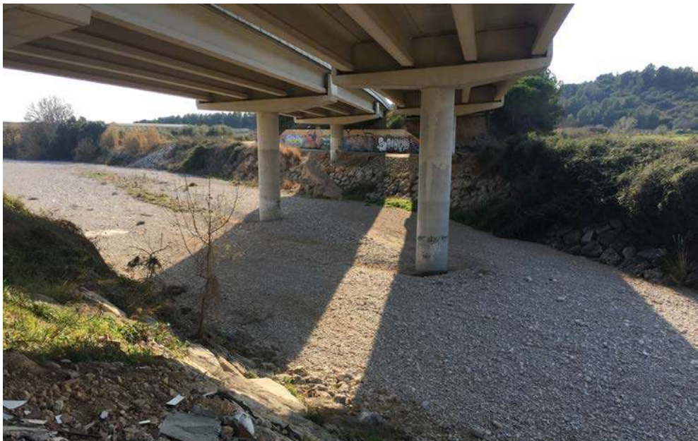
Figure 105. Bridge of the C32 over the Río Foix (Cubelles, Barcelona). The location of the pillars in the active channel could have been avoided.
