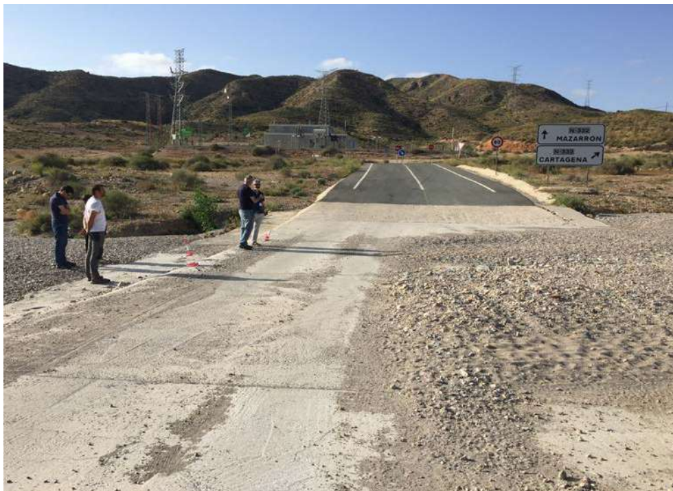
Figure 134. Ford built in a particularly active channel reach on the Rambla de Valdelentisco, next to Isla Plana (Cartagena). During the floods, a large bedload (sand and gravel) passes through this road-stream crossing, with the consequent danger that it represents for vehicle access.
