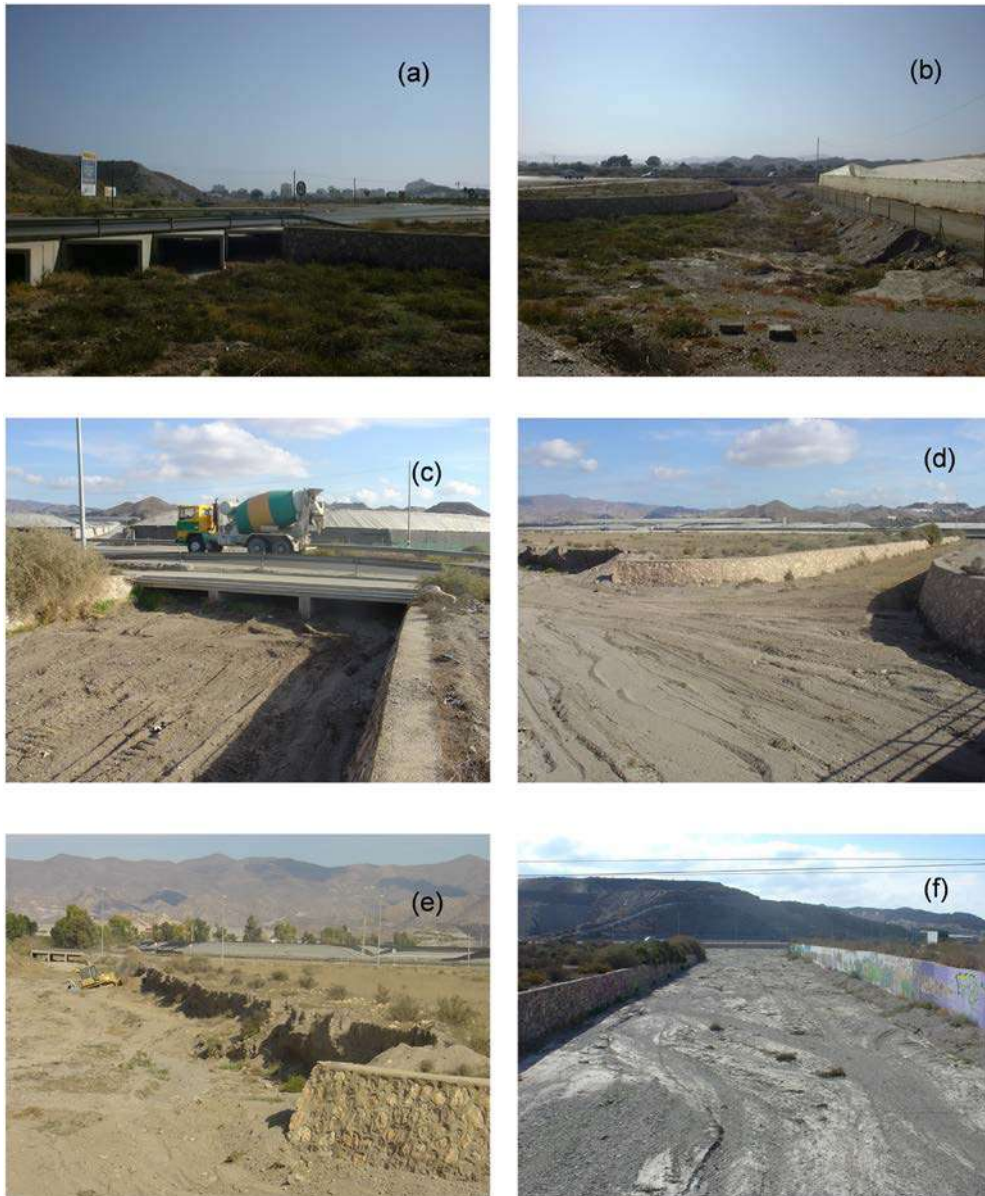
Figure 144. Ephemeral streams near Águilas (Murcia) with protective lining walls for greenhouses (a, b and c) located in the floodplain (even in the active channel), with narrowed channel reaches (a and b), promoting vertical bed accretion processes (d, e and f).
