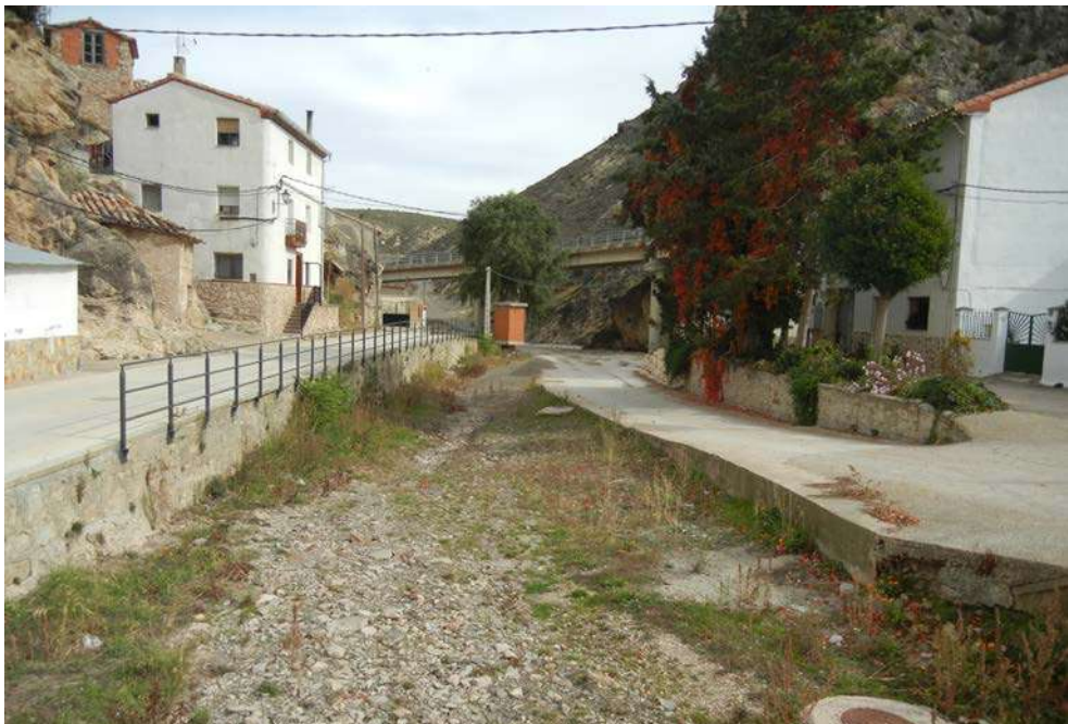
Figure 111. Pipes and collectors lead to a further narrowing of the Río Seco channel (Hoz de la Vieja, Teruel)
