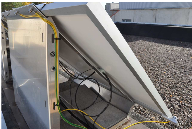
Figura 4.2. Platinum RTD attached to the back-side part of a PV module.
