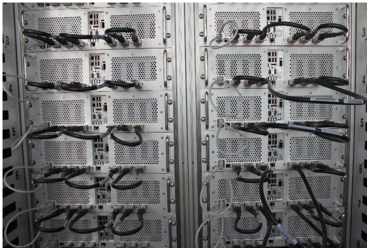
Figure 4: Close-up view of the Janus II machine installed at BIFI (Zaragoza). The installation has 16 Janus II boxes (12 are visible in the picture). The cables supporting the data-links in the z direction are mounted in loop-back mode for test purposes.
