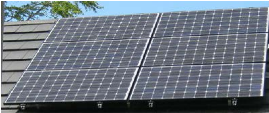
Figura 11. Panel solar fotovoltaico HIT [10]
