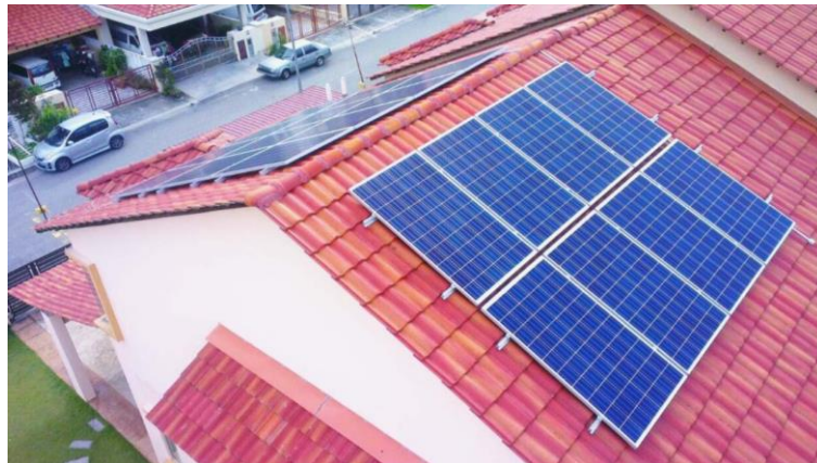
Figure 21: Example of solar PV system installation at residential unit
