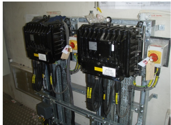
Figure 17 ID Fans Box Vane Dampers Electronic Panels
