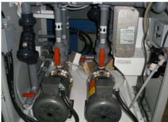
Figure XIV: VSD Primary Cooling System Pumps
