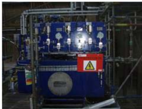
Figure X: ID Fan A Lubrication Oil Skid
