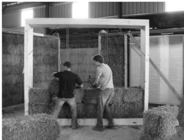
ILUSTRACIÓN 2. RECUPERADA DE: DEVELOPMENT AND TESTING OF A PROTOTYPE STRAW BALE HOUSE, KATHARINE WALL, PETE WALKER, CHRISTOPHER GROSS
