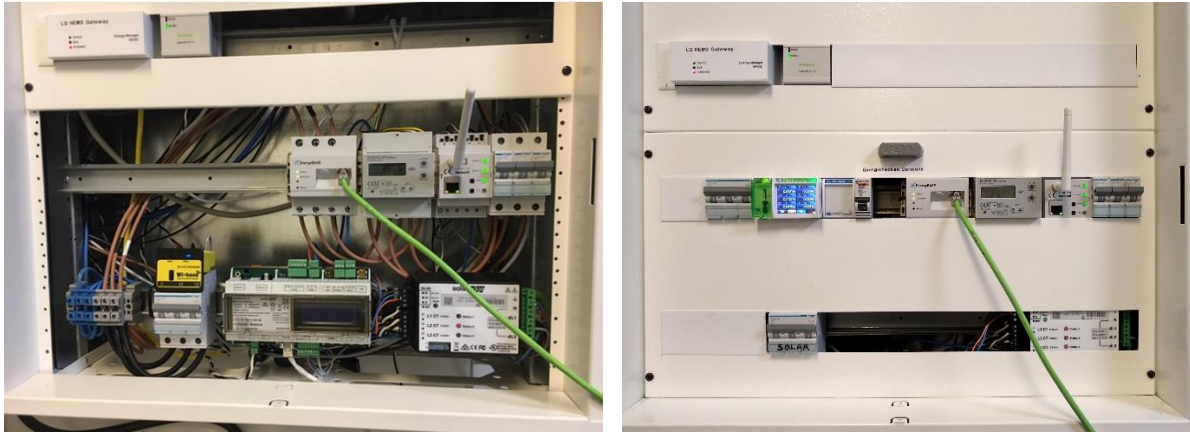
Fig. 14: Previous (left) and current (right) installation in the electricity room at Älvkarleby. Central left is the power meter PQube. Central middle is the communication box to receive reference solar cell (serial RS485 communication). Bottom right is the SolarEdge energy meter that communicates (sensors) to SolarEdge monitoring platform.
