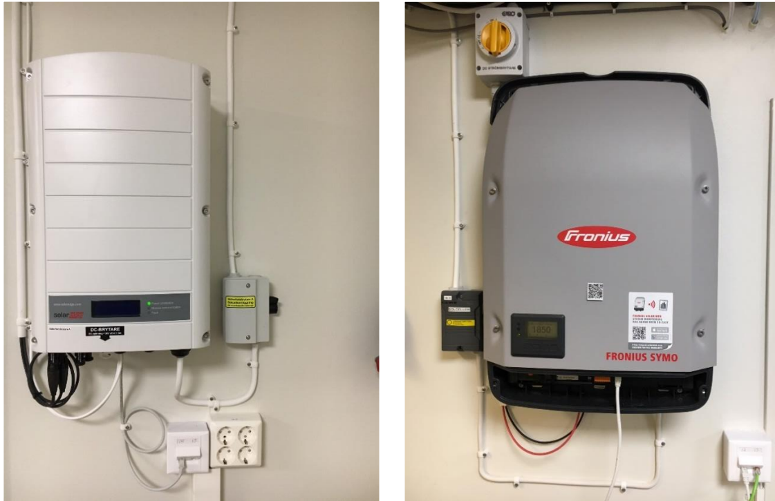
Fig. 12: Current installation of inverters in the electricity room at Älvkarleby: SolarEdge (left) and Fronius (right)
