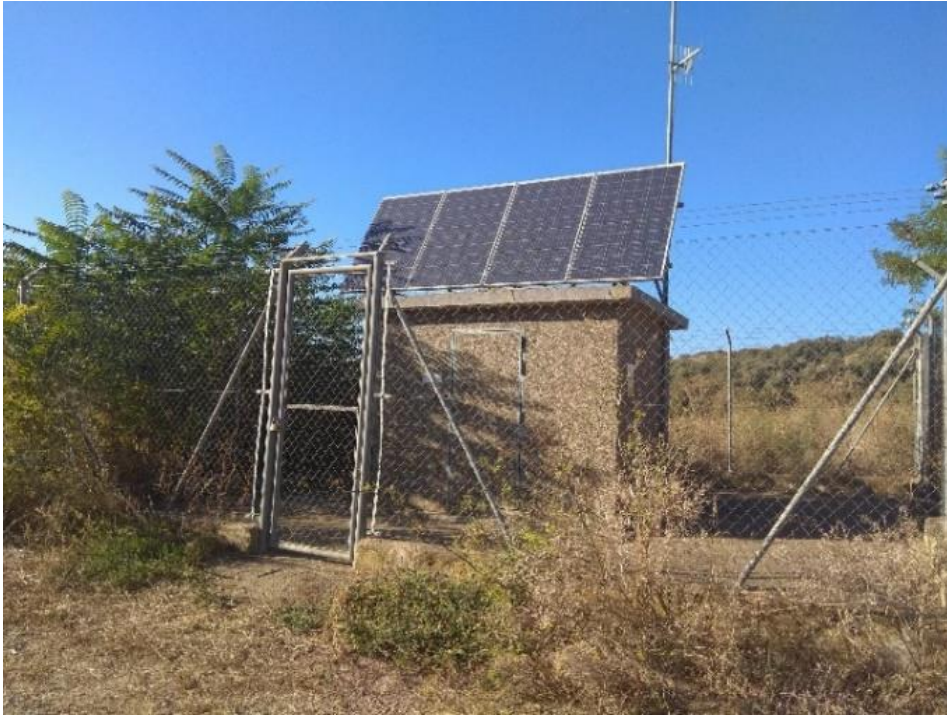
Figure 1. Standalone photovoltaic (PV) installation with metering and communication equipment.
